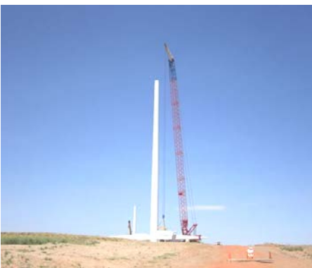
4. A tower is fully erected; the nacelle and rotor are being prepared for erection.
